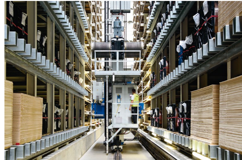
The implementation of the LTW stacker crane with a payload of 7.7 tons and a height of 29 meters takes place within the agreed time. Compared to the previous crane, amongst other things bigger cable drums and optimized cable guide ensure less bending and therefore a longer life expectancy of the cable.
