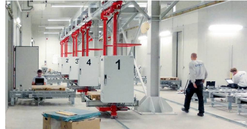
Integration of an electric monorail system (EMS) by the LTW team. The main advantage of the EMS lies in the scalability – in case of a prospective expansion, vehicles can easily be added, during reduced system operation disengaged, for repair purposes separately moved into the climatized maintenance area.
