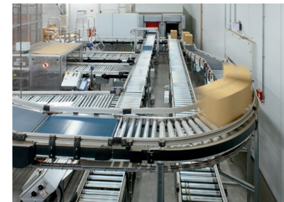
The automated small parts warehouse and the conveyor connection to the order picking area are designed for a plurality of different container sizes and qualities.
